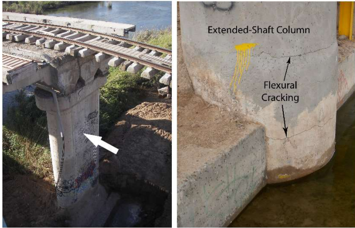
Fig. 3. Railroad bridge collapse due to pier translation in direction of arrow (left; photo D. Murbach) and flexural cracking of highway bridge columns in response to lateral spreading (right).
