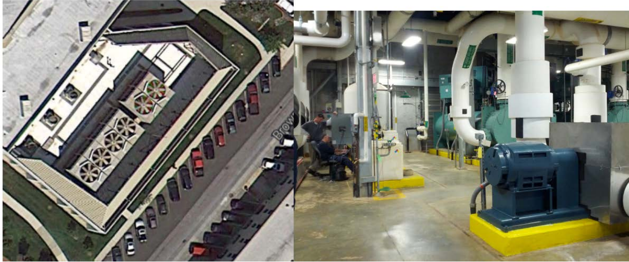
Figure 15. Lejeune plant cooling towers (left), chillers and pump (right)
