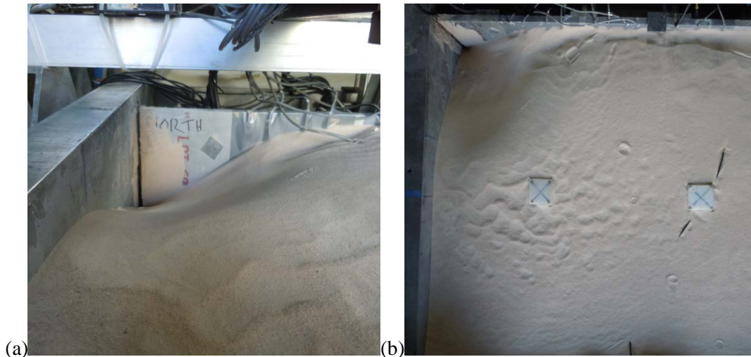
Figure 3.13: Cave in at northeast corner of structure
