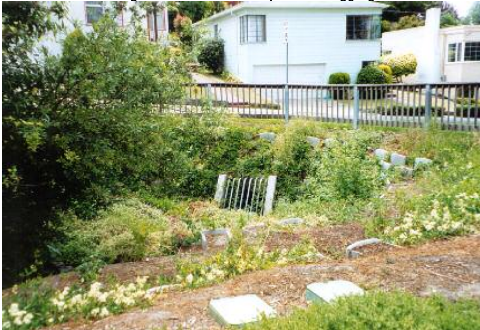
Figure 4. Photo of downstream inlet of Baxter Creek in Poinsett Park. Notice small retention basin constructed and grate over the inlet to prevent clogging from trash and debris.
