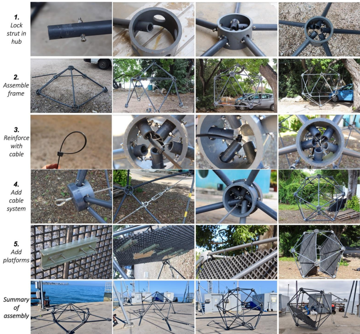
Figure S2.25 Assembly of Two-Platform Ark framework. Struts are inserted into hubs and locked into place via bolts and locknuts, and then a stainless-steel wire rope is passed through the finished structure to increase the strength. Two platforms are then added, bisecting the Ark horizontally.
