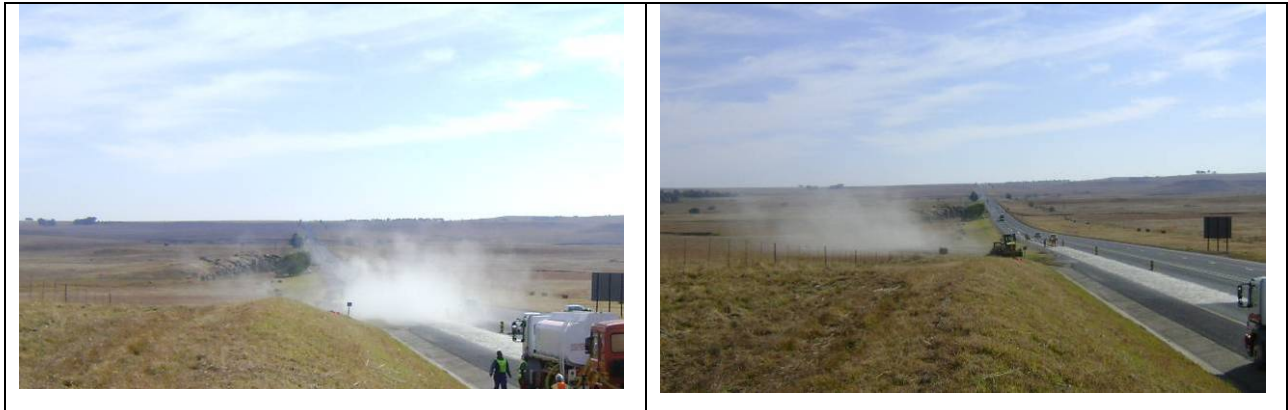
Figure 7.2: Cement loss by wind.
