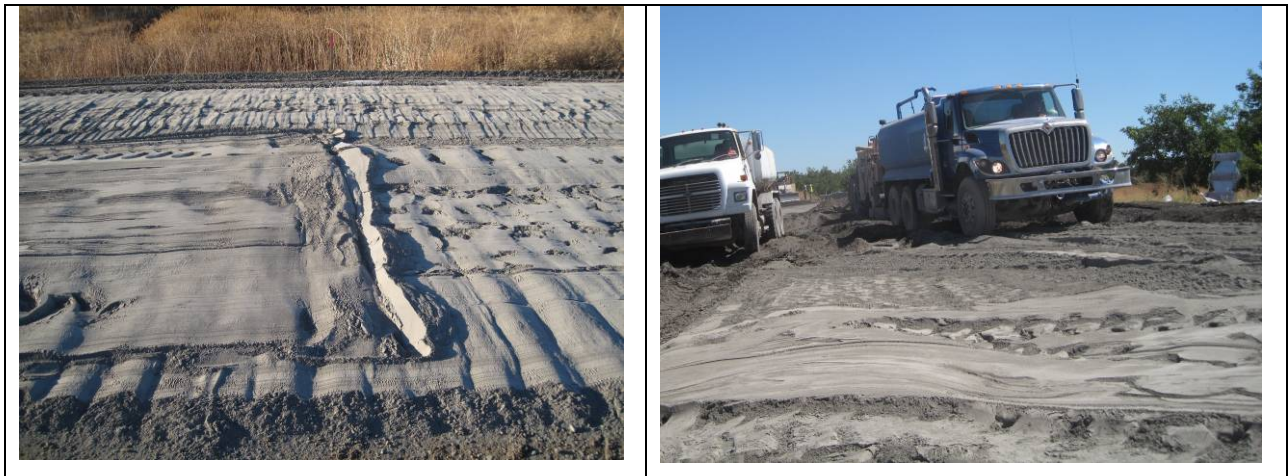
Figure 7.3: Uneven distribution of stabilizer on road surface.
