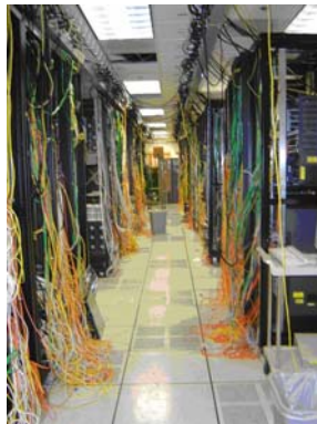
Figure 1 Typical computer rack lineup in the data center
