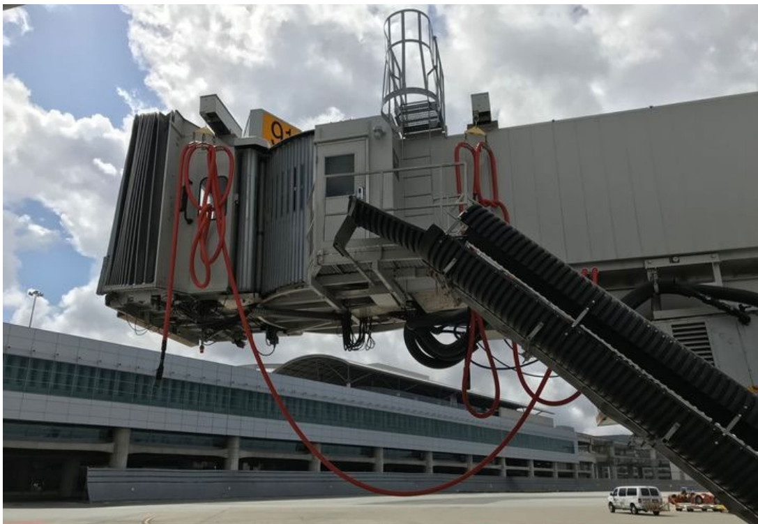
Figure 30: Jet bridge with GP cable connected to a pulley system at SFO international airport (Achatz Antonelli, 2019)
