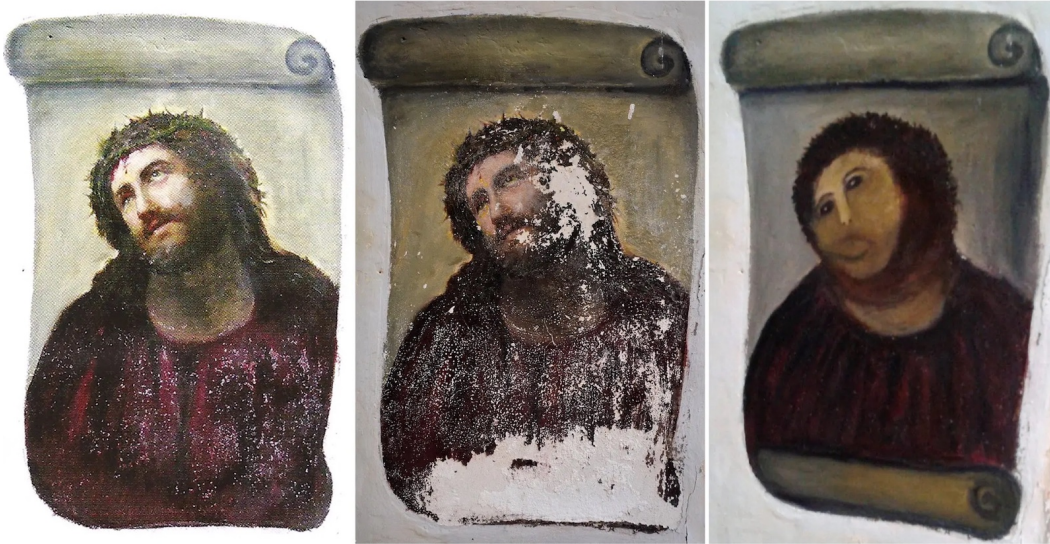
Figure 2.3. The botched 2012 “restoration” of Elías García Martínez’s 1930 fresco, Ecce Homo , located inside Mercy Church in Borja, Spain
