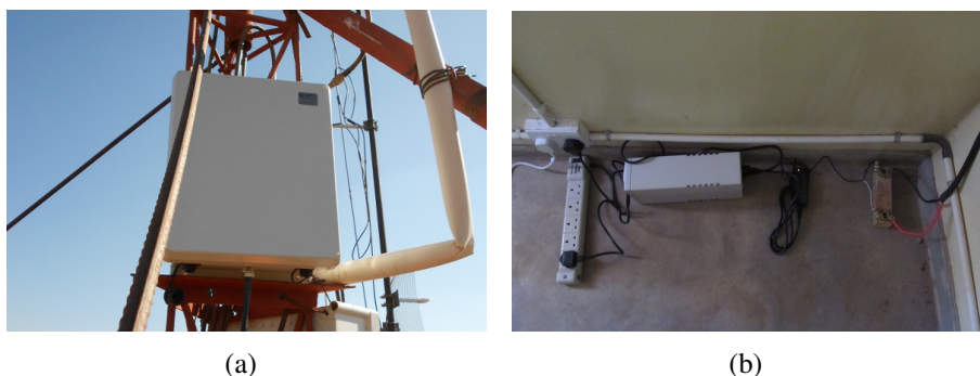
Figure 6.5: Our equipment in Macha: (a) the base station and (b) the power supply.
