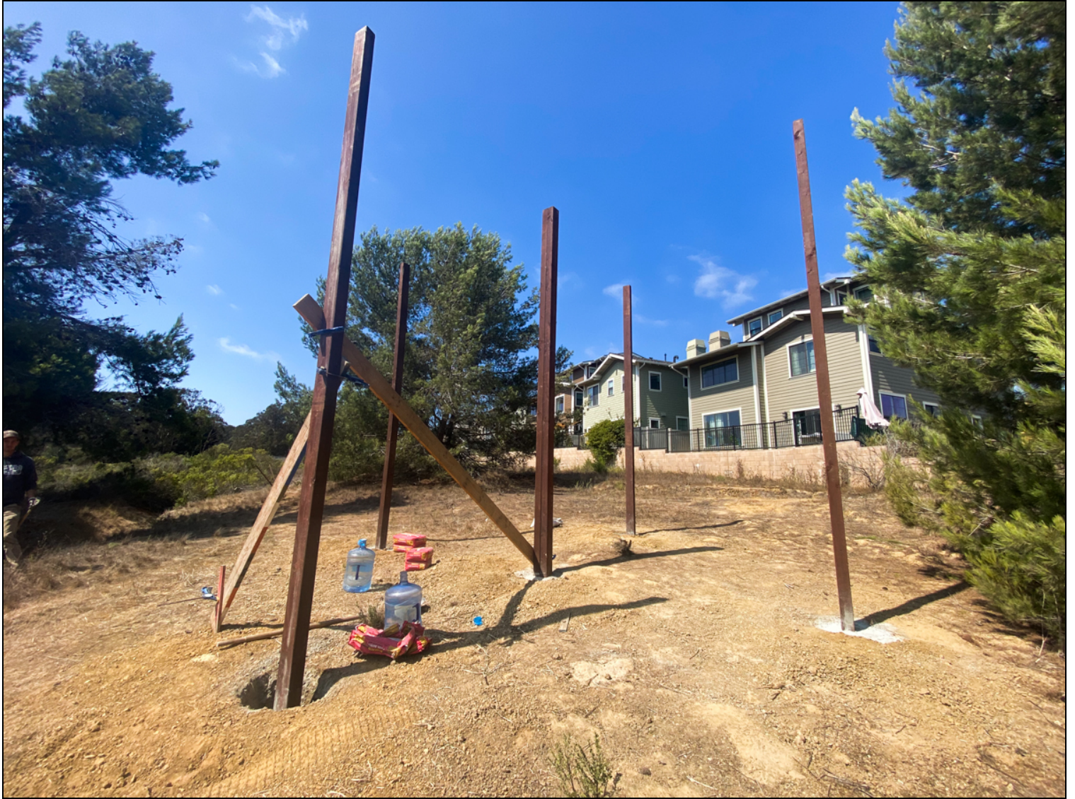
Construction begins! These posts will support the nesting structure as seen in the photo below.
