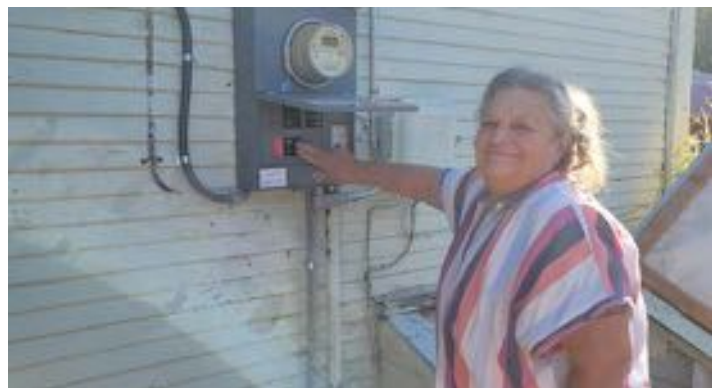
Patricia Barrett flips the switch to turn on new GRID Alternatives solar panels on her home. Photo credit: Patricia Barrett
