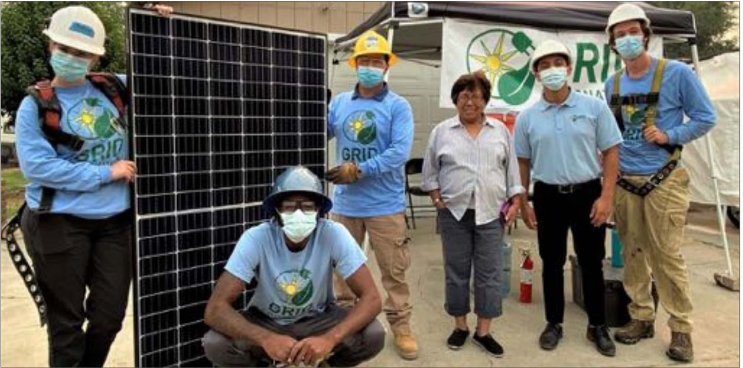
GRID Alternatives staff and trainees install rooftop solar PV panels in the TCC project area. Photo credit: GRID Alternatives
