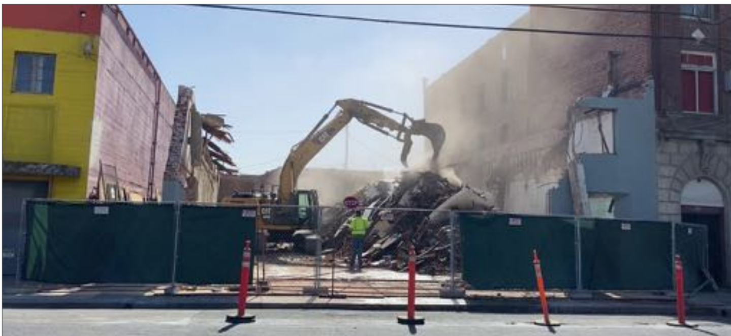
Demolition of Rrazil Social Cub, a culturally significant building in Stockton’s historic Little Manila district, after financing could not be secured for structural repairs. Photo credit: Little Manila Rising
