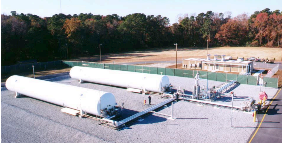
Figure 58 Northstar Industries City Gate LNG Plant
