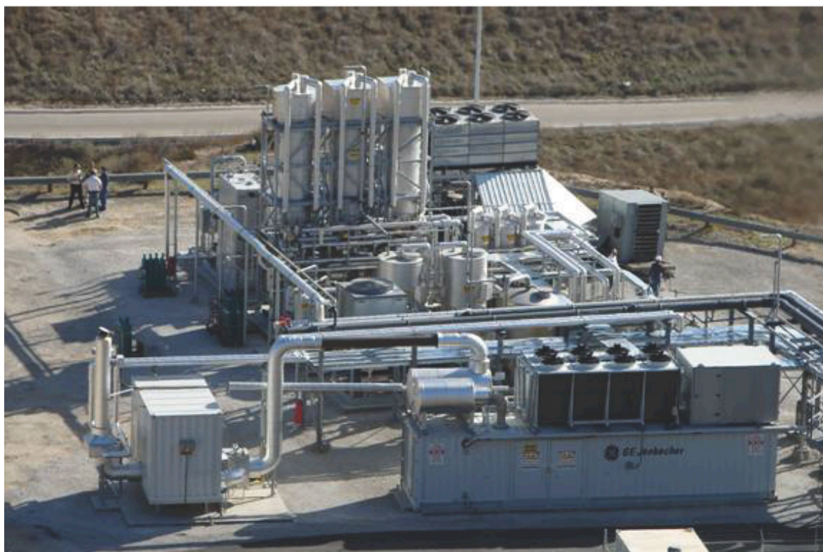
Figure 55 Prometheus Commercial LNG from Landfill Gas Facility
