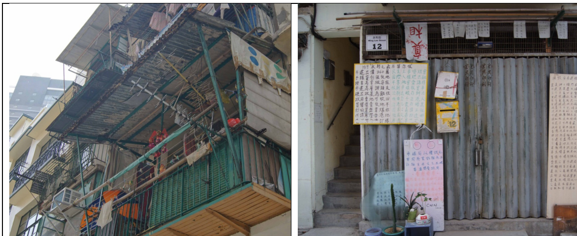
Figure 4.9 The ruined environmental condition of buildings in Wing Lee Street (photos were taken in 2013 during renovation).
