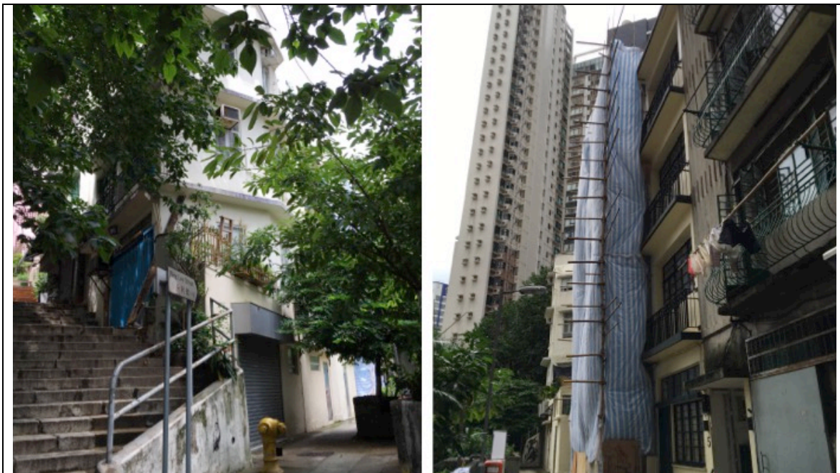
Figure 4.11 Wing Lee Street in 2016. Most of the buildings have been renovated and are being used by the charities. Only some of them were still under construction.
