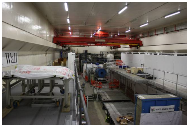
Figure 6: View of the MICE Hall, looking upstream. The wall separating the Hall from the ISIS vault is in the background of the photo, and the final quadrupole (blue) of the muon beam line is in the center. All of the remaining MICE components will be installed downstream of the quadrupole and upstream of the muon beam dump visible in the foreground.
