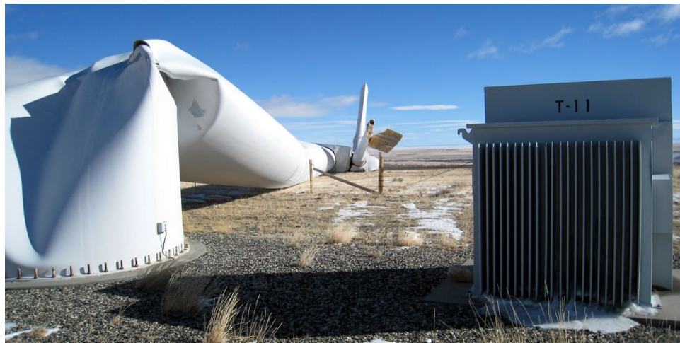
Figure 1.2: Collapse of a wind turbine at the Foote Creek Rim wind energy facility near Arlington, in Wyoming, USA, in 2010.
