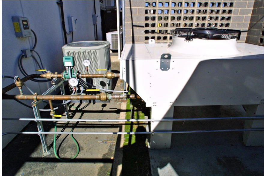
Figure 4-3: Dry Cooler Outside of NRL Data Center
