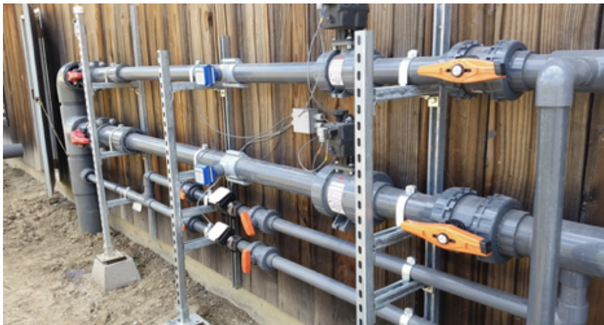
Supplemental Figure 1. The plumbing manifold for the Porter Creek augmentation structure.
