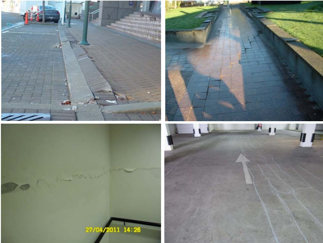
Figure 5.6. Post-Christchurch earthquake photographs of Building C: (upper-left) rolling of curb outside of building indicated area of cyclic softening-induced ground movement; (upper-right) deformation in tiled walkway and planter walls on west side of building above basement; (lower-left) cracking of wall in north corner stairway to car park; and (lower-right) cracking of garage basement RC mat (from CCC)
