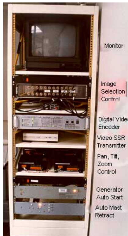
(b) Right equipment rack
