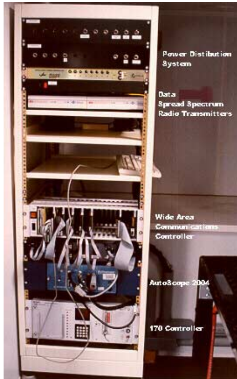
(a) Left equipment rack
