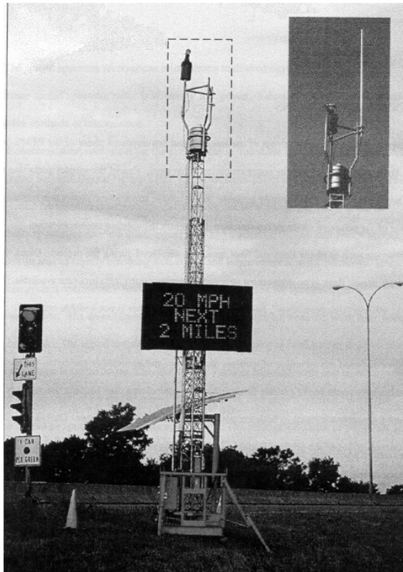
Figure 1-8. PTMS deployed on a skid
