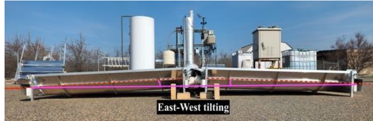
Figure 7. 3 The images show the main system components, two modules with six vacuum glass tubes, a hot water tank, and other system components. The lower photo has a line added to emphasize the small tilt used to shed rainwater. These photos were captured on Feb 10 th , 2023, at 10:19 AM after about 447 days of operation.
