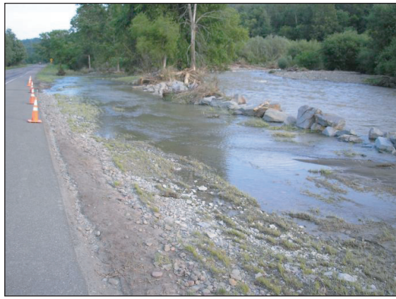
Figure 8. Canasawacta Creek is undermining Route 23. This is where the creek was moved from the north side of the road to its present location. Flooding occurs often in this location.
