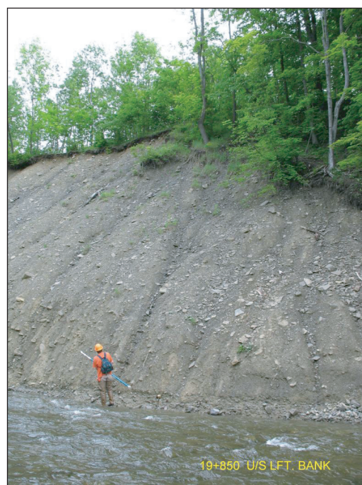
Figure 5. Eroding south bank of Canasawacta Creek just upstream of the Moon Hill Road bridge. Material is continually sloughing off into the creek.
