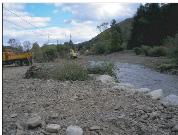
Figure 13. The bench provides an area for high water between the creek and Route 23. The willows were planted and they are doing quite well. The utility pole is not shown but the bench protects it from the creek.
