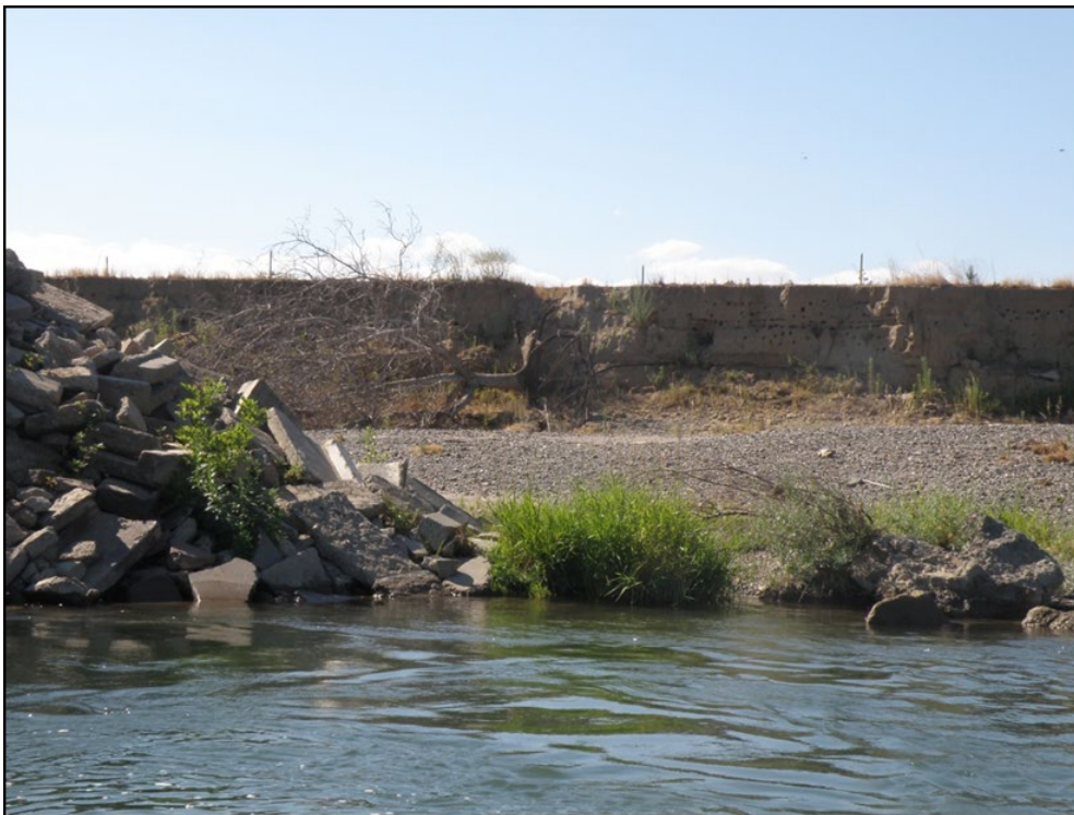
Figure 3.1. (Top) Plan view of private landowner-installed rock revetment failure at River Mile 186 with Bank Swallow colony on the cut bank behind the failure, Butte County, Sacramento River. (Bottom) Burrows on the bank which has eroded behind the alignment of failed revetment.
