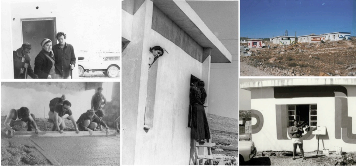
Figure 2.5 Settlement activists renovate the military barracks (Etzion on the right in the two images on the left). Source: Ofra Archive.
