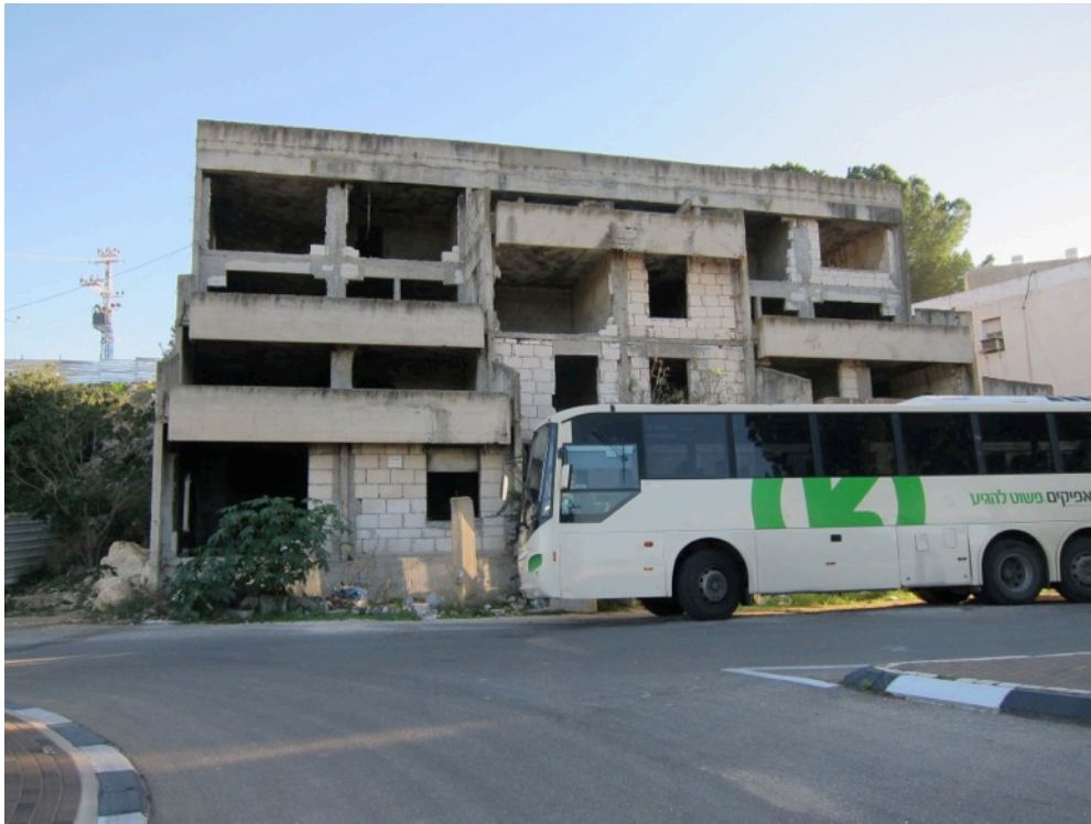
Figure 4.12 Abandoned houses in Immanuel. Once construction had stopped, many of the housing compounds in Immanuel were left in different stages of construction. The vast majority of them have remained abandoned. Photo by author.
