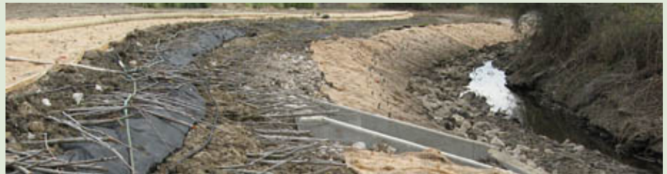
Soon after the banks of El Encanto Creek (Phelps Ditch) were laid back, willow cuttings and erosion control blanket were installed as part of the restoration and bank stabilization project.
