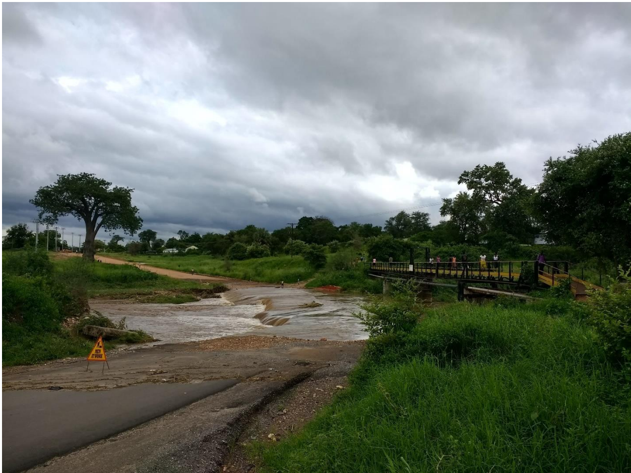
Photograph 6: A flooded vehicle road with adjacent pedestrian bridge. Hhaala Collieries, Southern Province, Zambia.
