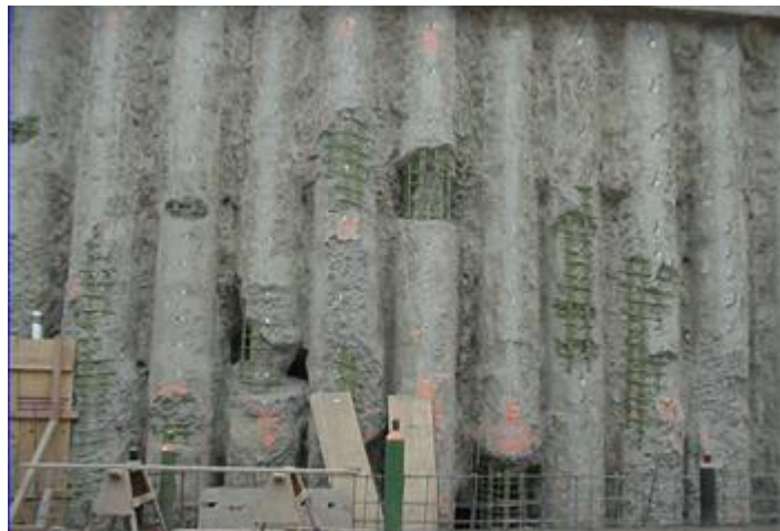
Figure 1-2 Air pockets in drilled shafts (Photo copyright: Dan Brown)
