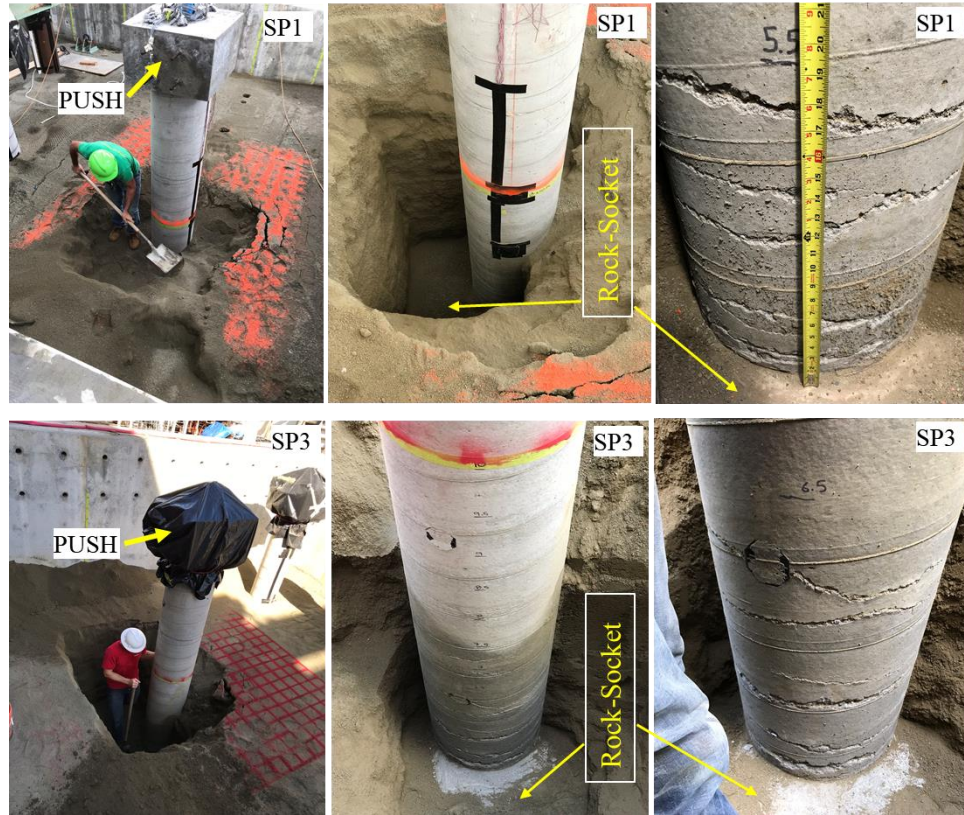
Figure 6-9 Crack pattern observation upon excavation of specimens 1 and 3
