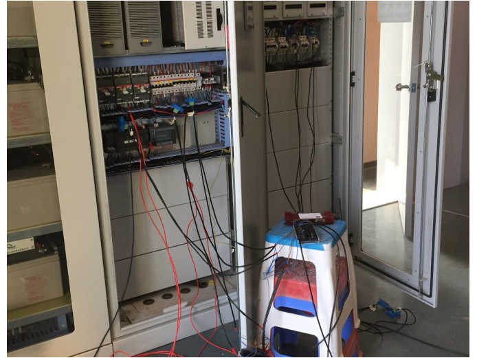
Fig. 5: A prototyped metering setup within the electrical cabinet of the DC Lab.
