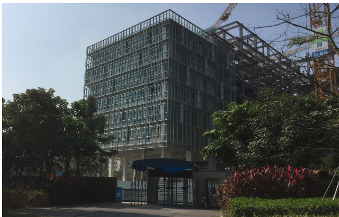
Fig. 6: The IBR DC office building, under construction at the time of the photo.
