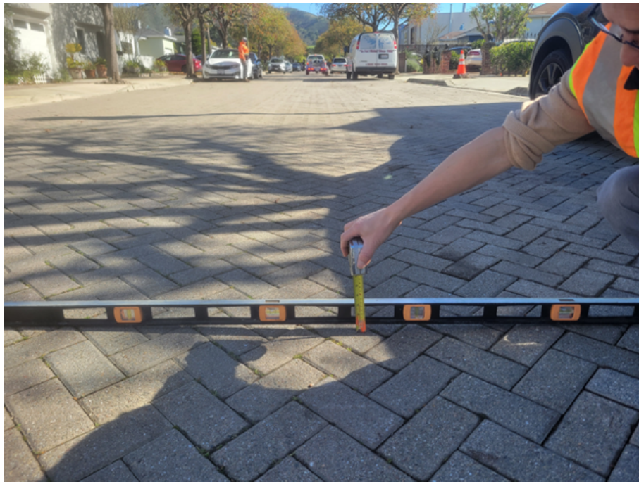
Figure 3.10: An area with some rut on the eastbound direction of the F Street at the Colma site.
