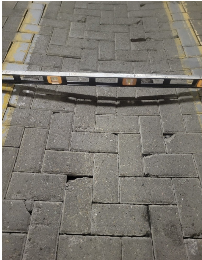
Figure 3.21: Example of a deep rut and damaged blocks in the gantry lane at the Port of Oakland near Berth 55.
