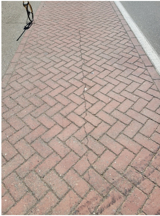
Figure 3.9: A longitudinal crack in the ICP-looking shoulder at the Capay site. (The asphalt shoulder was stamped into paver shape.)
