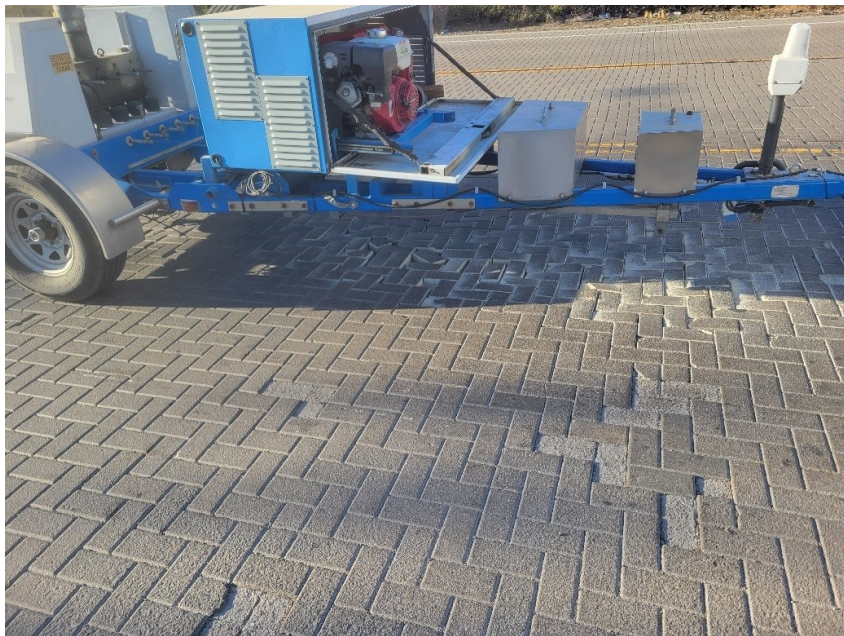
Figure 3.18: An area with extensive rutting and paver damage in the ICP at the Westley site.
