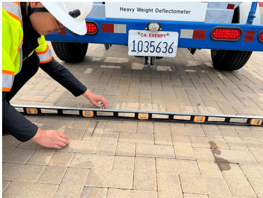
Figure 3.16: A section with more than 10 mm (barely noticeable) rut at the Rancho Cordova site.
