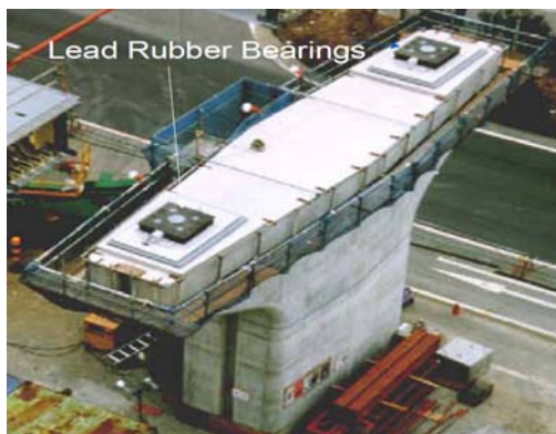
(a) Lead rubber bearings used on Fukae Viaduct after 1995 Kobe earthquake
