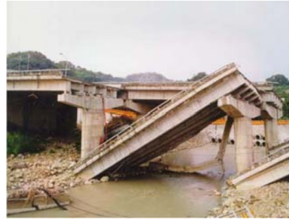
(b) Unseating failure during the 1999 Chi-Chi earthquake
