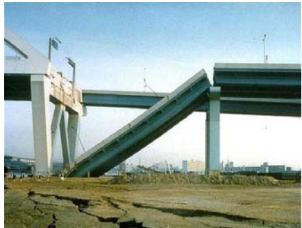
(g) Span collapse of the Nishinomiya Bridge following the 1995 Kobe earthquake
