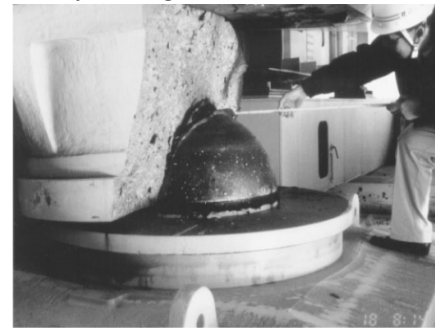
(f) Bearing failure during the 1995 Kobe earthquake.
