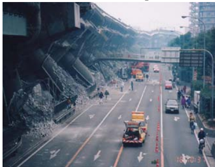
(e) Column flexural failure during the 1995 Kobe earthquake.
