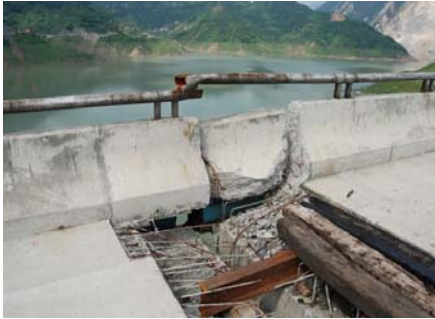
(a) Expansion Joint Damage during the 2008 Wenchuan earthquake
