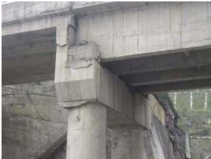
(c) Retaining block damage during the 2008 Wenchuan earthquake
