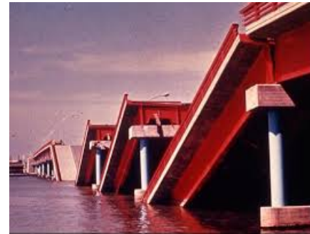
(h) Span collapse and pier failure of the Showa Bridge in the 1964 Niigata earthquake
