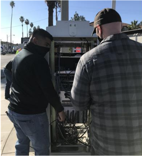
(a) At Traffic Controller Cabinet
