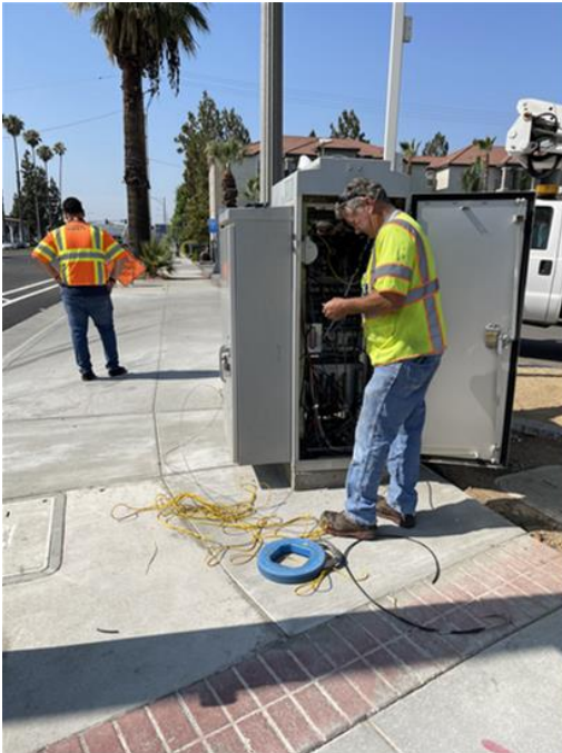
(a) At Traffic Controller Cabinet
