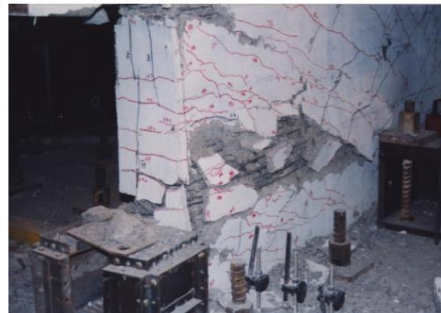
e. Damage at wall base (end of test)
