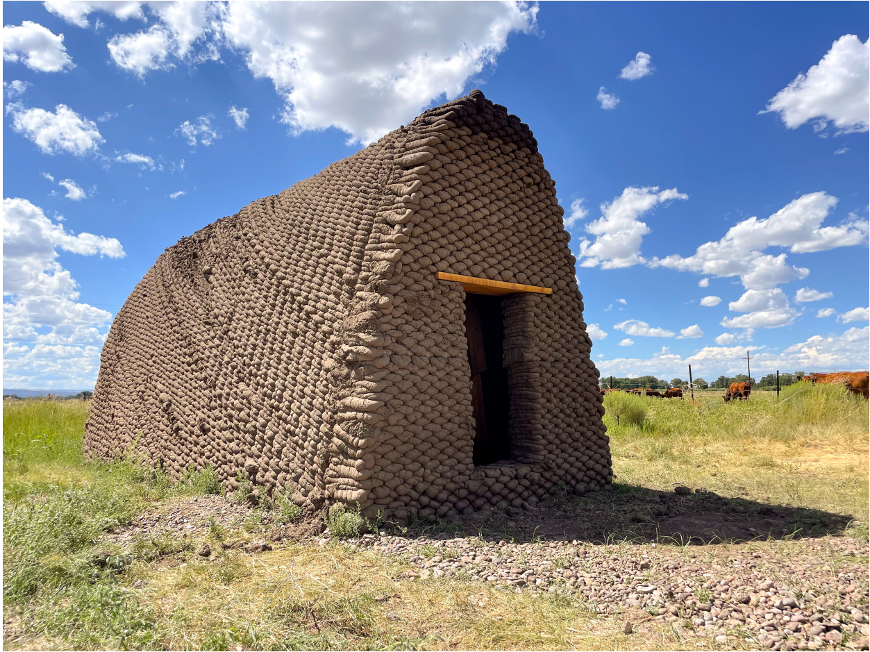
Figure 7.14: Front view of the completed formwork-free, 3D-printed Nubian vault made of adobe.
