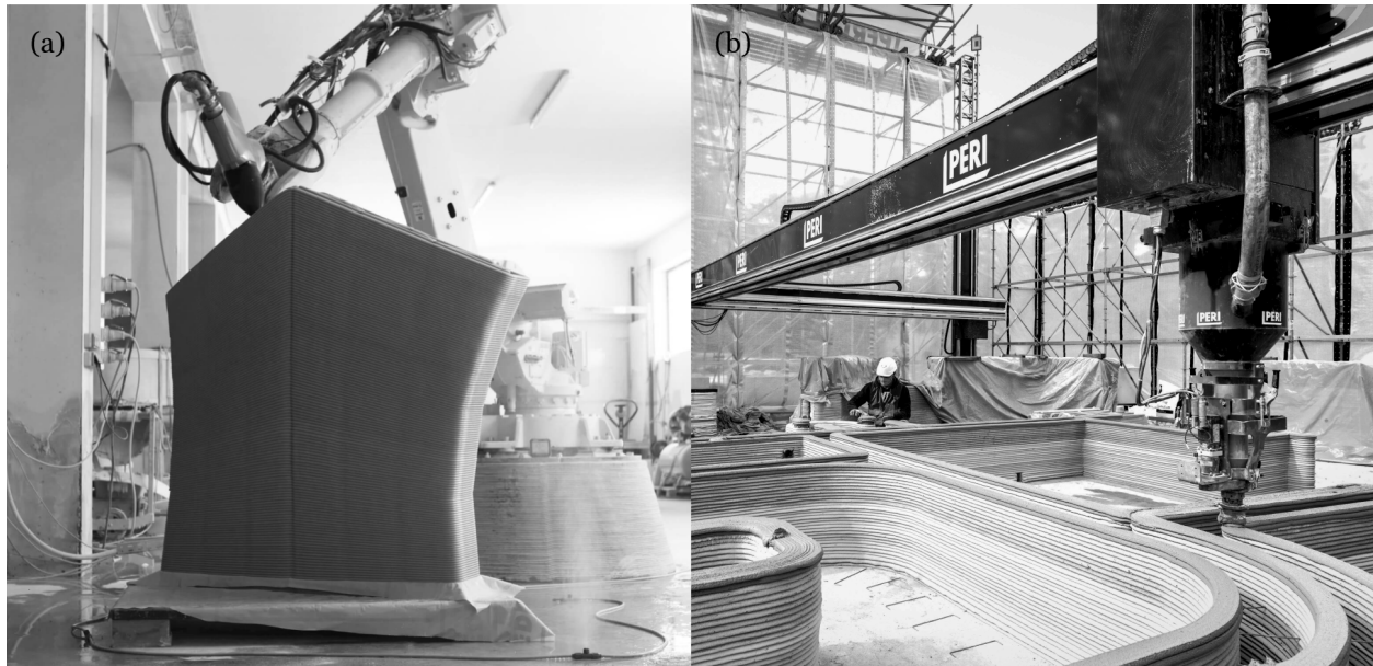
Figure 2.5: Comparing additive construction processes. (a) 3D printing prefabricated concrete components using an industrial robotic arm [115]. (b) In-situ construction 3D printing, featuring the BOD2 gantry-style 3D printer [120].
