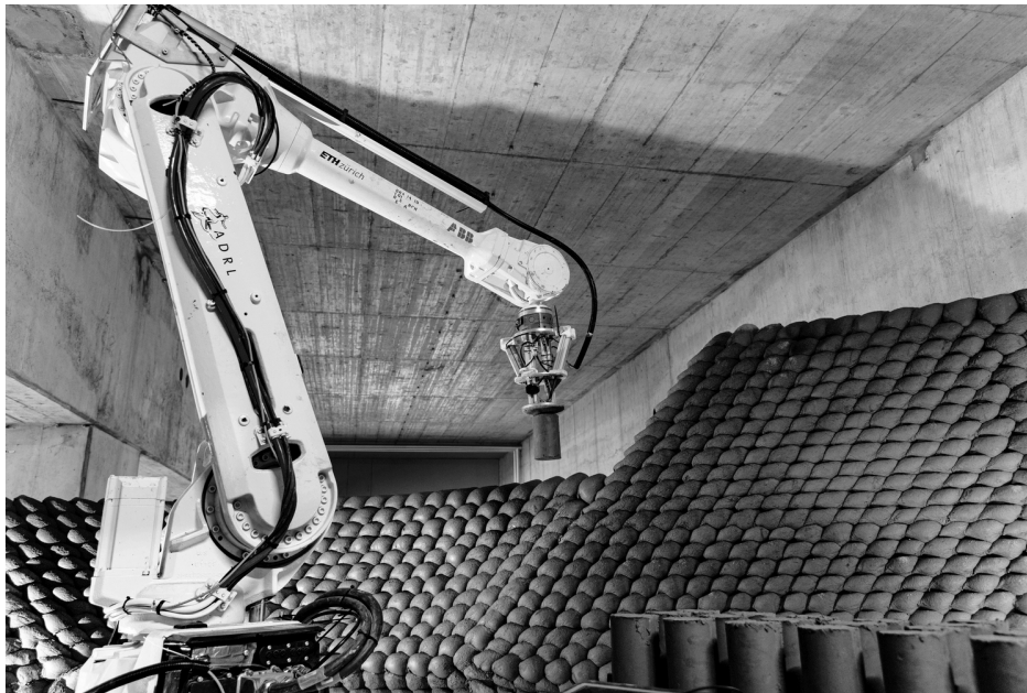
Figure 2.6: Example of a creative application of industrial robotic arms in architecture, demonstrated by Gramazio Kohler Research, ETH Zurich, in their Clay Rotunda project [250].
