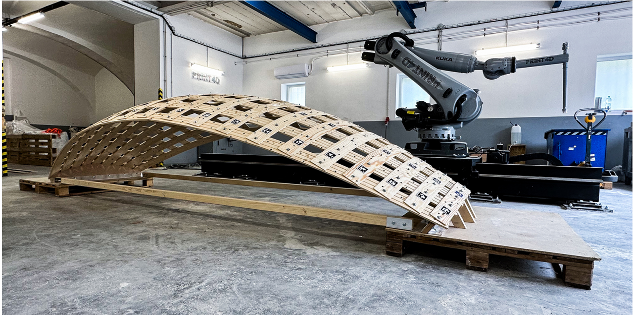
Figure 5.7: The finished bending-active formwork was made of 9 longitudinal and 22 transverse timber strips and fitted with fiducial markers to facilitate registration of the exact formwork geometry.
