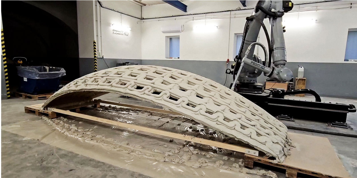
Figure 5.12: Multiple layers of concrete are 3D printed onto a lost, bending-active formwork to create a wide-span, material-efficient hybrid gridshell.
