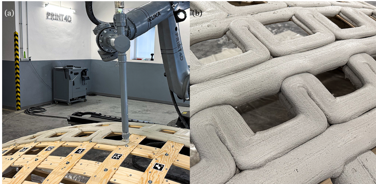
Figure 5.11: Conformal 3D printing process on bending-active formwork in action. The multi-axis printing platform ensures that the concrete is distributed evenly with a constant layer height and that the nozzle maintains a normal orientation to the formwork.
