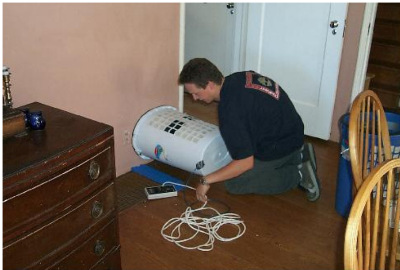
Figure B8. Residential supply airflow measurement
