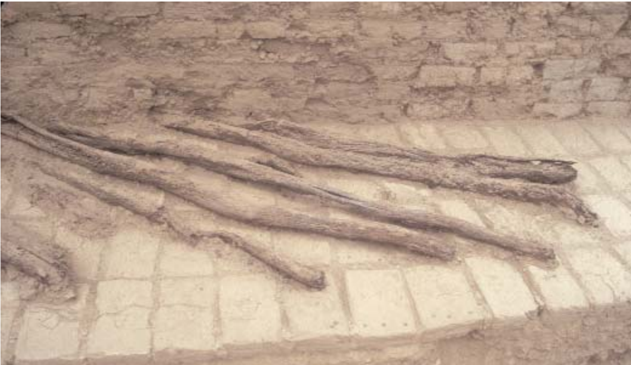
Figure 4.18 Wood beams were placed diagonally over the adobes above Tomb B to prevent the new construction from slumping under the weight of the solid adobe masonry that was being added to fill the South Room.
