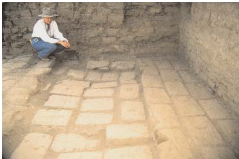
Figure 7.2 Adobes slumping above the burial chamber of Tomb 1.
