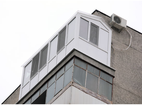
Fig. 13 Balcony enclosures using the thermopane enclosure system. A practice often found in the post-socialist era
