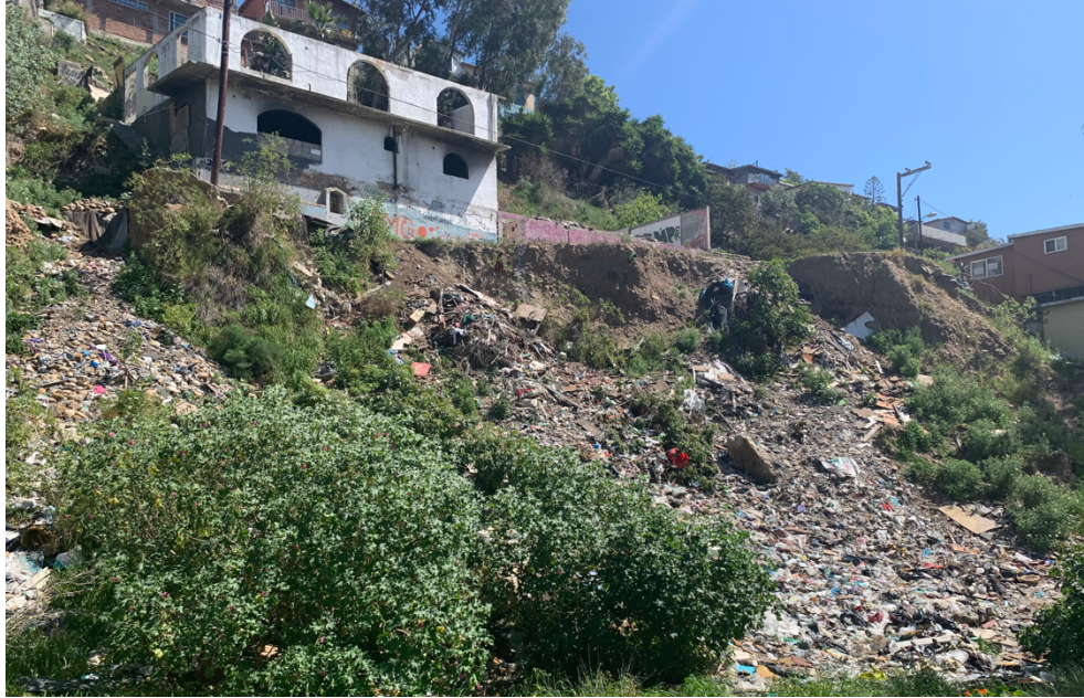
Figure 8. Photo of Anexa Miramar displaying the site of a major landslide that occurred in 2015 with many homes destroyed and residents displaced. The area succumbed to an erosion event. Source: Photo taken by Natalia Rangel.
