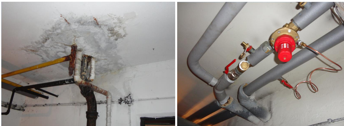
Figure 4.5 Condition of the heating system piping in the original (left) and the renovated (right) buildings (Source: Author)
