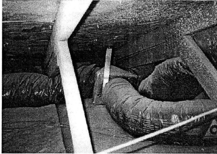
Figure 4. New plastic flexible ducts in an attic
