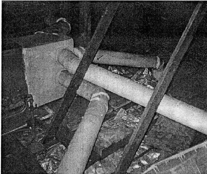
Figure 3. Asbestos insulated sheet metal ducts in an attic
