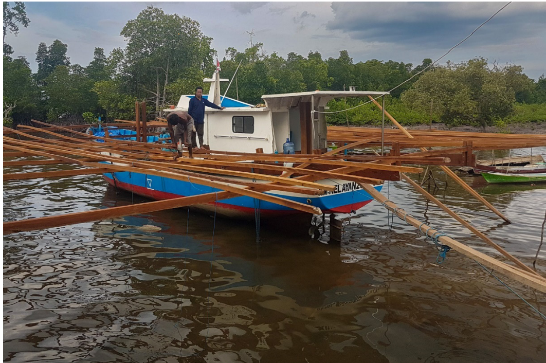
Figure 21 (top): A bagang in Laikatahi | Figure 22 (bottom): A new bagang under construction, framing over a boat aquired with government aid.
