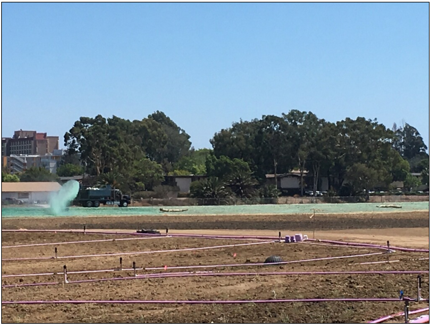
Sterile wheat hydro-mulch being sprayed to help stabilize slopes during the coming winter rains.
