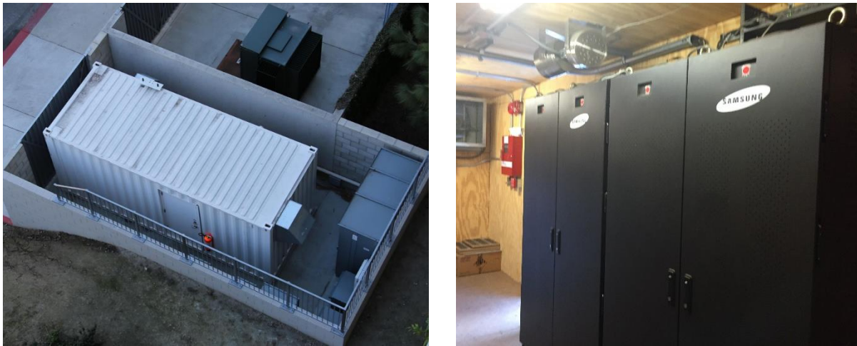
Figure 9: Battery Energy Storage System Enclosure (left) and Samsung cells (right)
