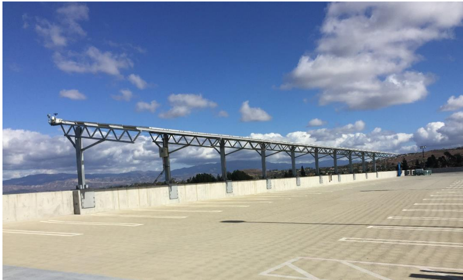
Figure 11: Anteater Parking Structure rooftop solar PV
