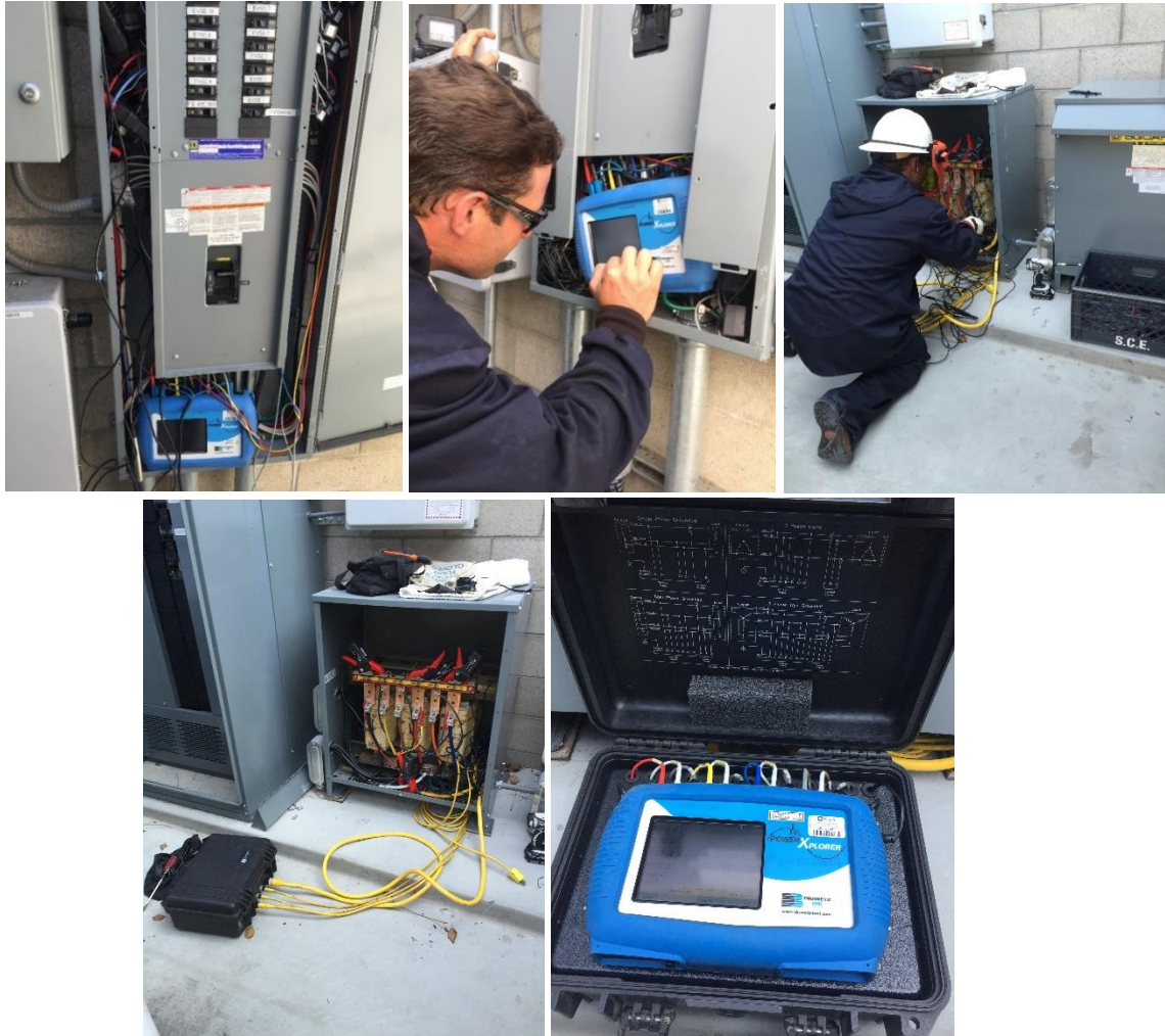
Figure 73: Power quality equipment installation by SCE Field Engineer.
