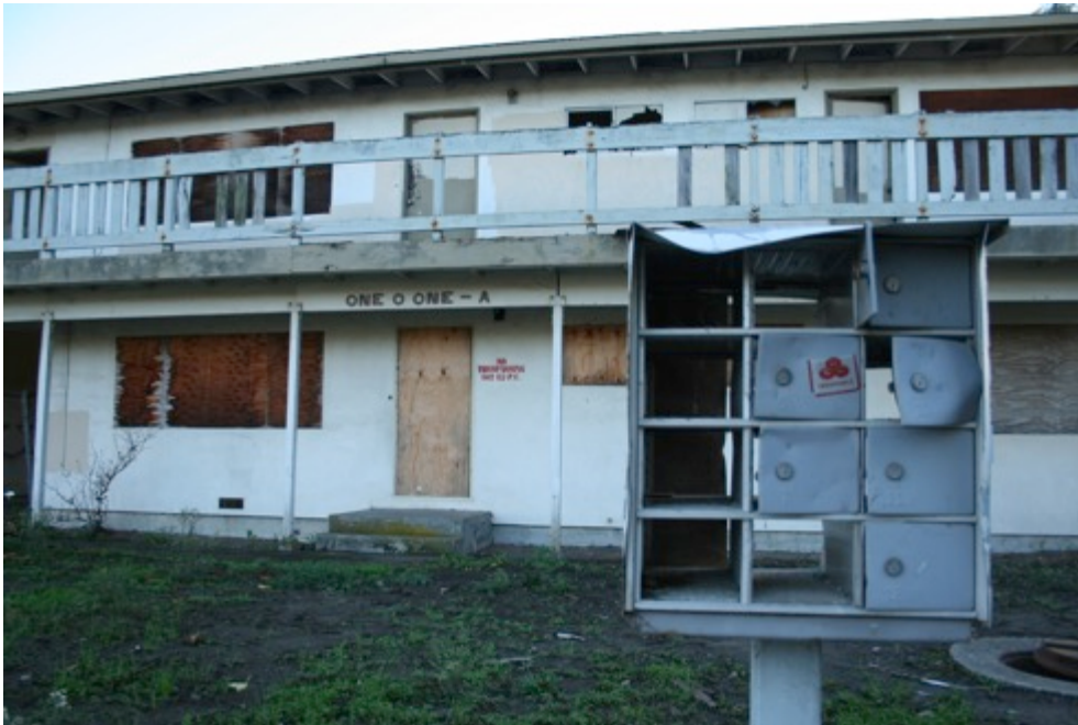
Figure 22: Alameda Point has decaying apartments that sit uninhabited. (Author)
