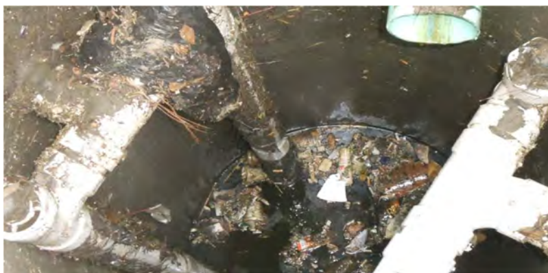
Photo of the primary chamber of a percolation well after a storm event.
