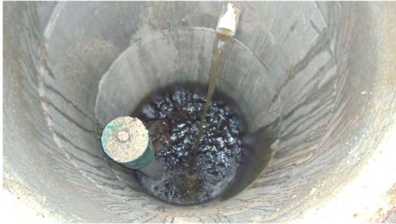
Photo of the secondary chamber of a percolation well after a storm event.
