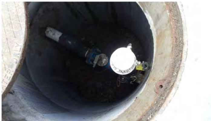
Photograph shows the piping for the flow meter between primary and secondary chambers to calculate the stormwater flow into the dry wells.
