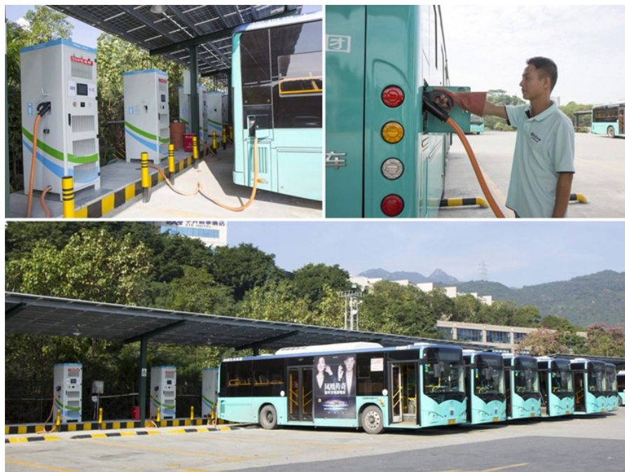
Figure 3-12 Liuyue Charging station operated by Winline
