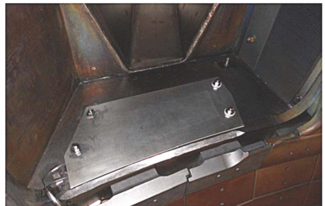
Figure 9. Molybdenum plate in vessel port box.
