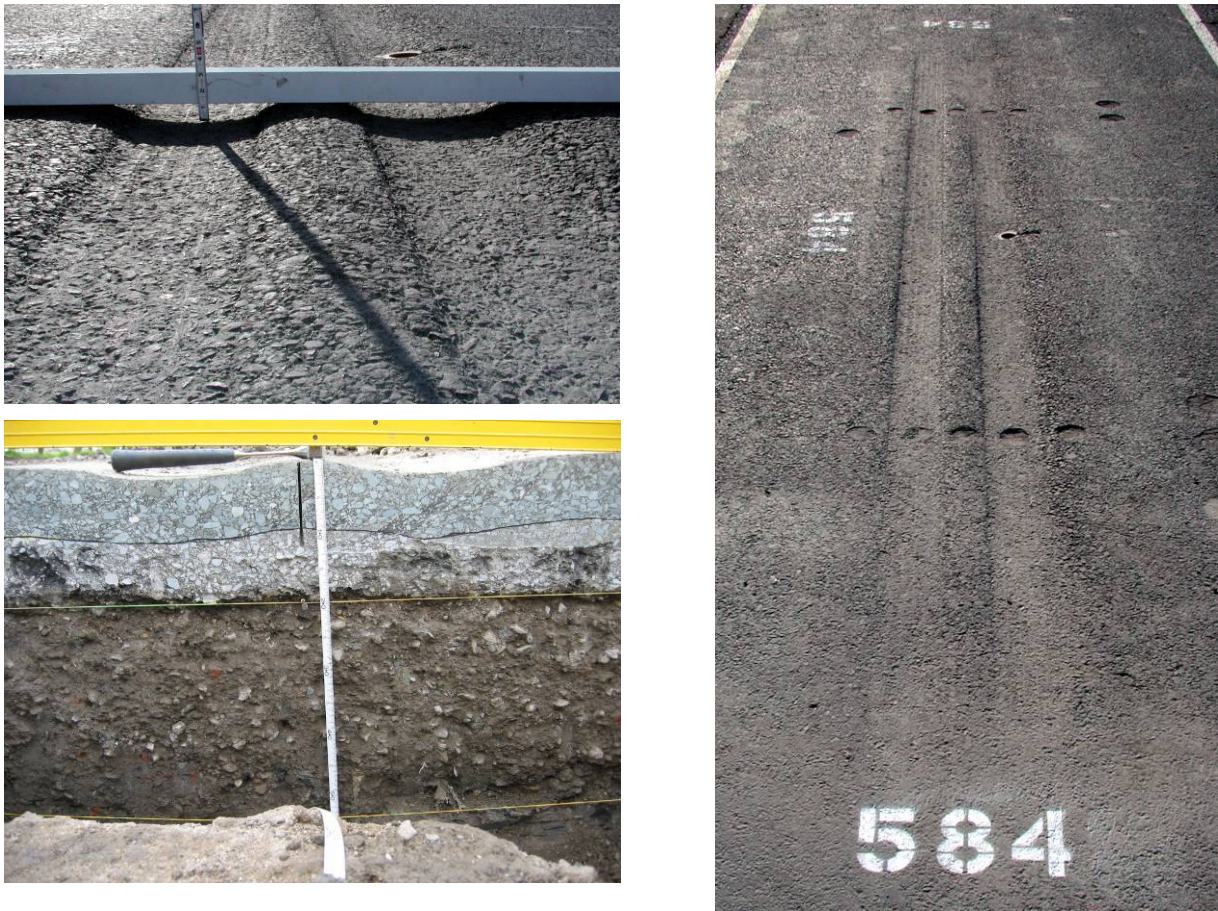
Figure 3.57: 584RF: Section photographs at the end of the test.
