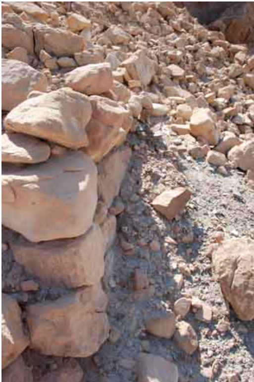
Figure 3.68: A wall at the top of the tailing pile, which may have surrounded a shaft entrance that is now covered with collapse.
