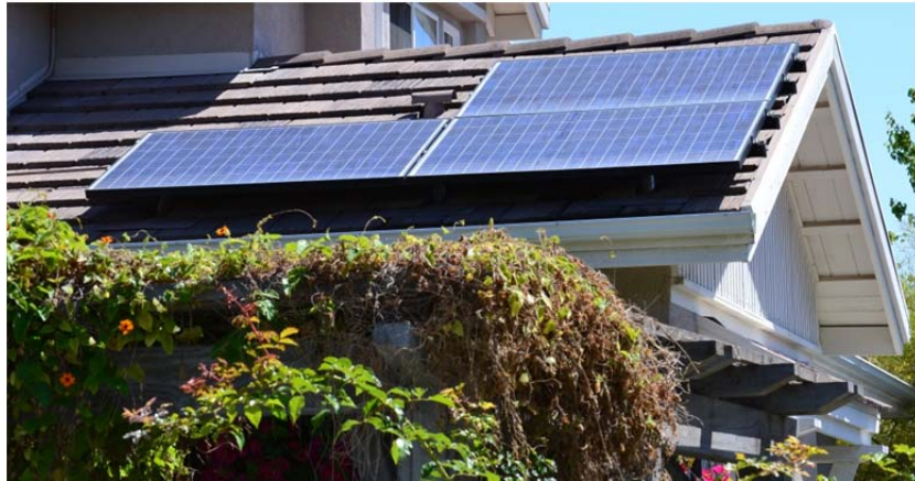
Figure 7. Solar panels installed at a residence
