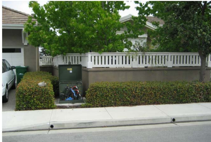
Figure 6. Padmount, single-phase, three wire secondary distribution transformer with open cover to show measurement equipment
