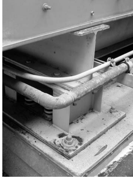
Figure A.4: Chiller support
