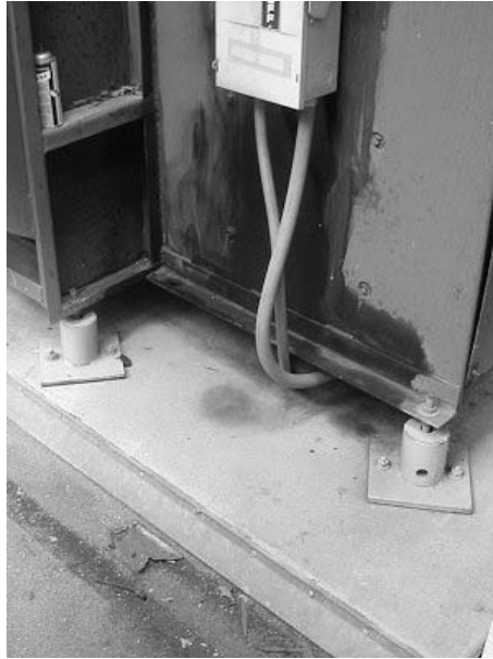
Figure A.3: Rooftop cabinet support
