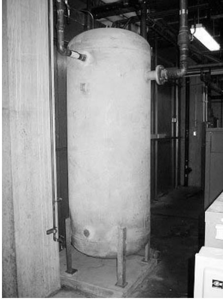
Figure A.9: Vertically oriented tank
